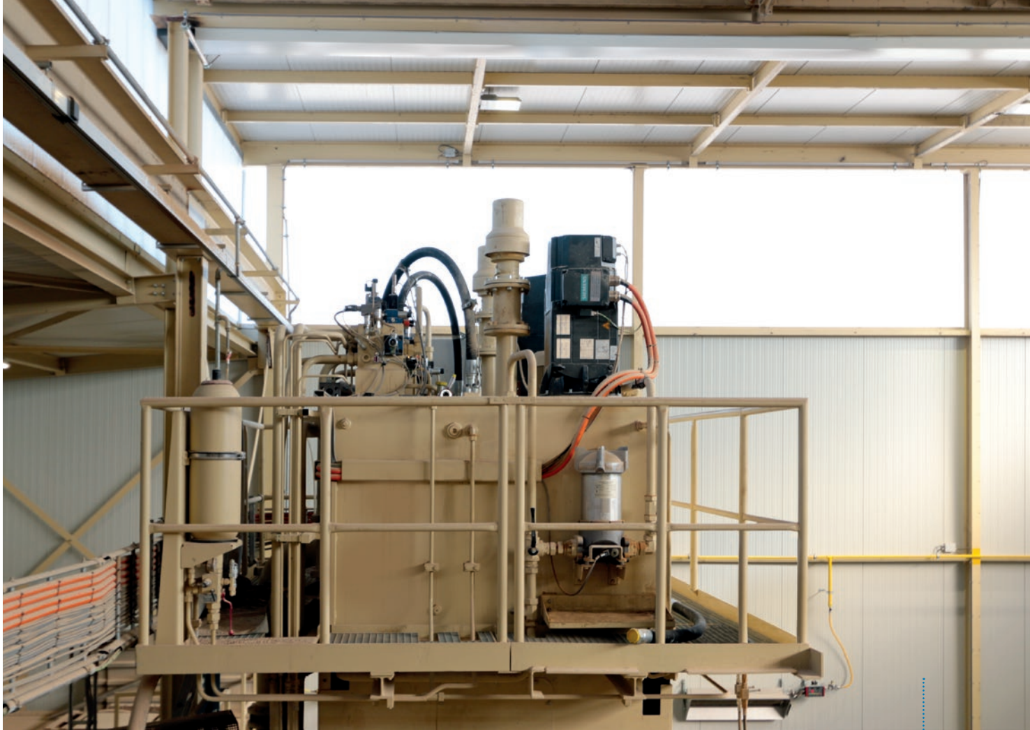
Mechanical drive system for servo hydraulics.
