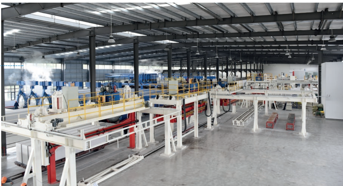
General overview of the plant.
