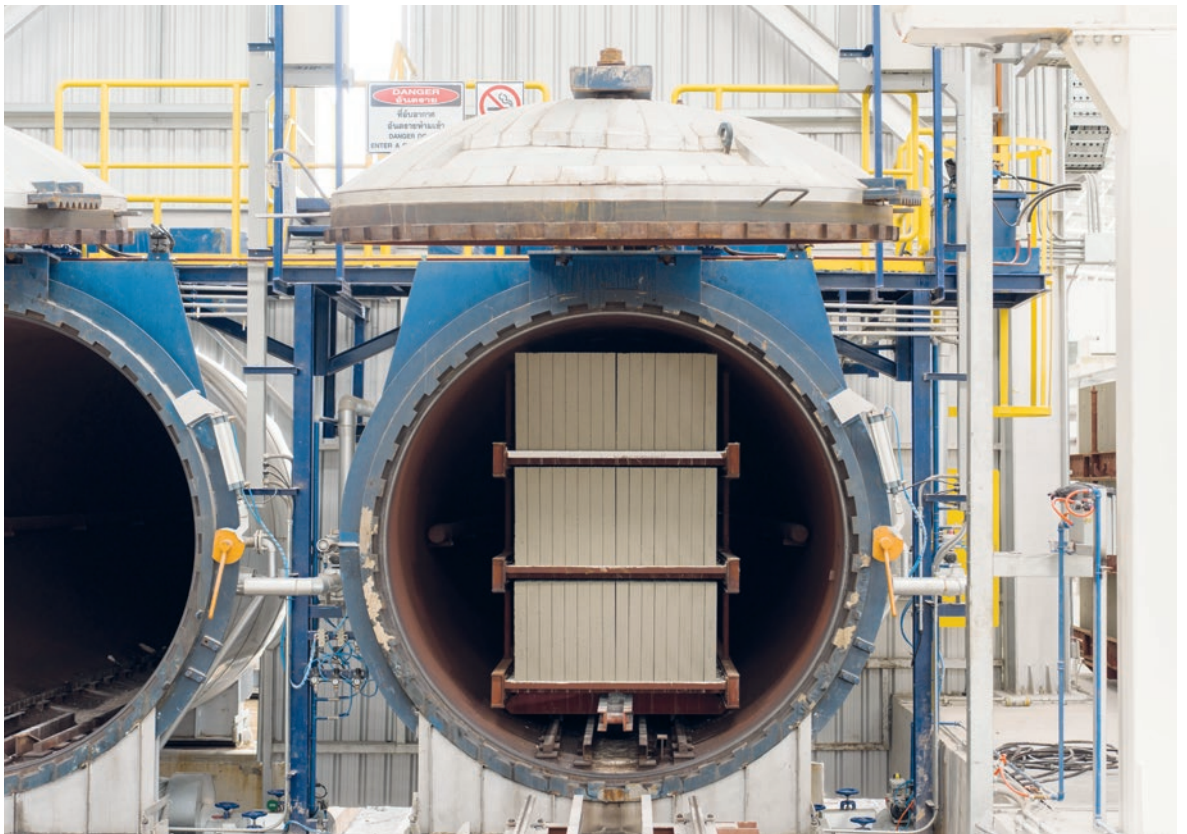
Flat cake autoclaving is one of the key technologies for producing thin AAC elements in the new Thai AAC plant.
