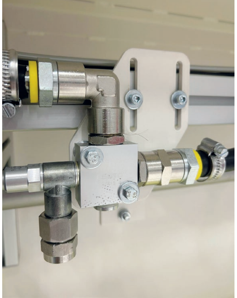
Fig. 4: Detail of the oil distribution manifold used for precise oil pressure spraying inside the mould.
