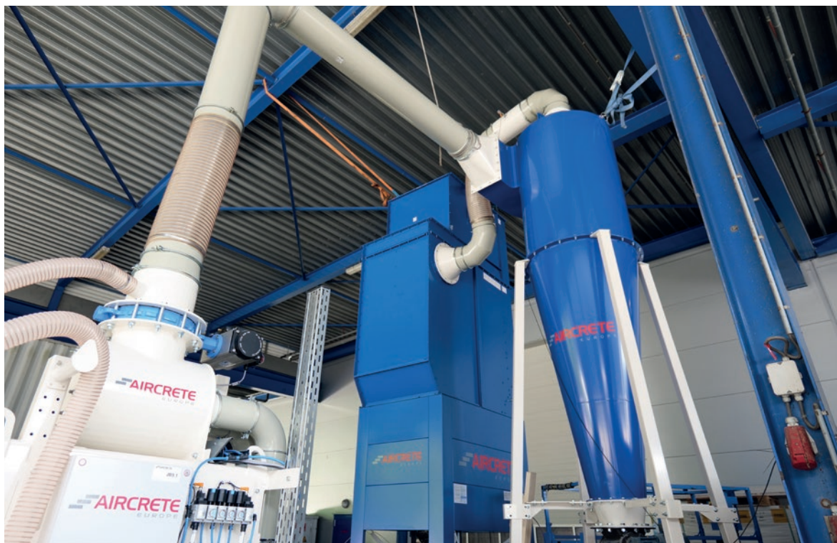
Cyclone-based dust collection system integrated into the U-block machine
